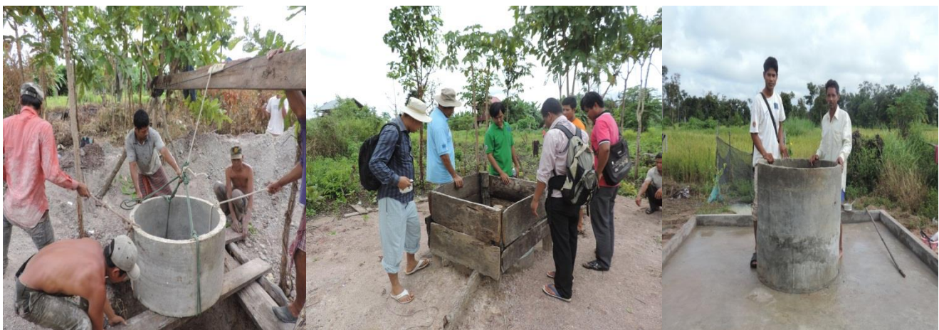
Process of ring well construction (left), Monitoring by project staff(middle) A successfully built ring well (right)
